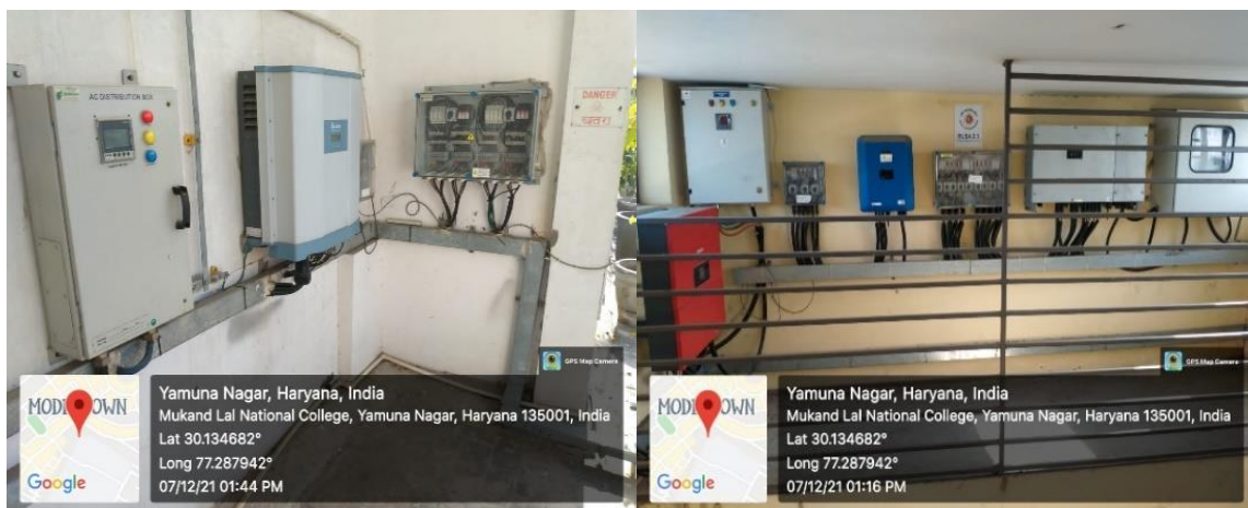
Solar inverters connected to grid for energy savings.
