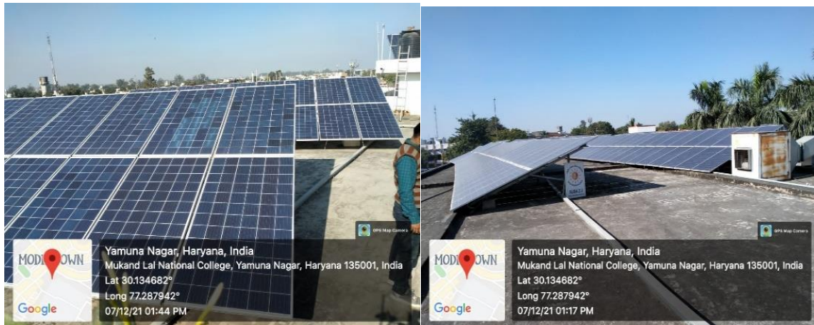
Solar Panels installed on the rooftop.
