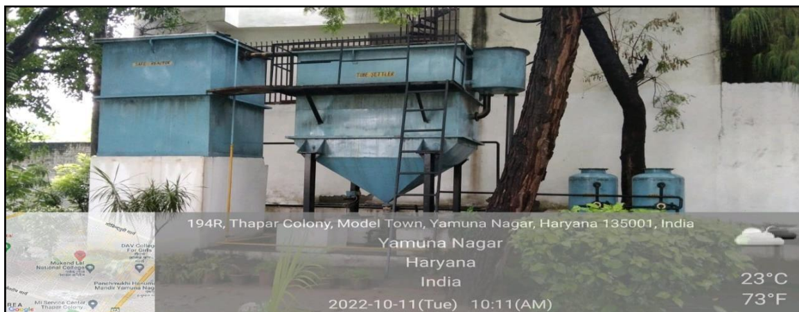
Photo of STP Plant
