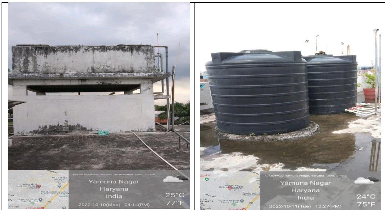
Fig: - 2.4 Water storage tank in college campus
