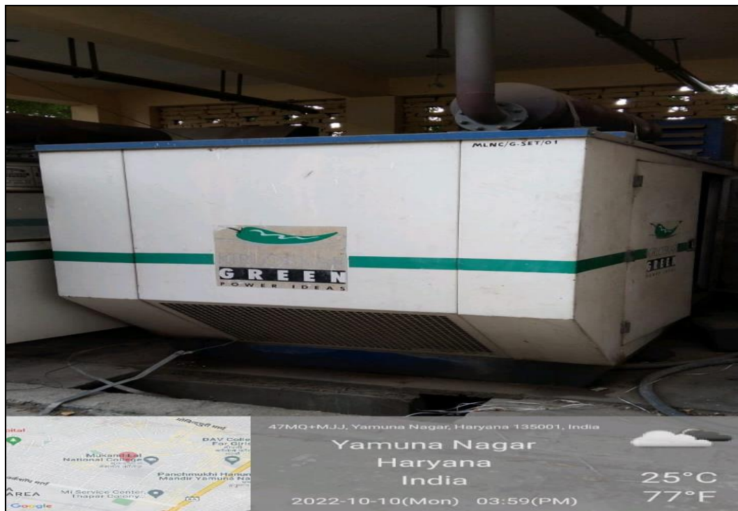
Figure 2.3:- DG set in Power House
